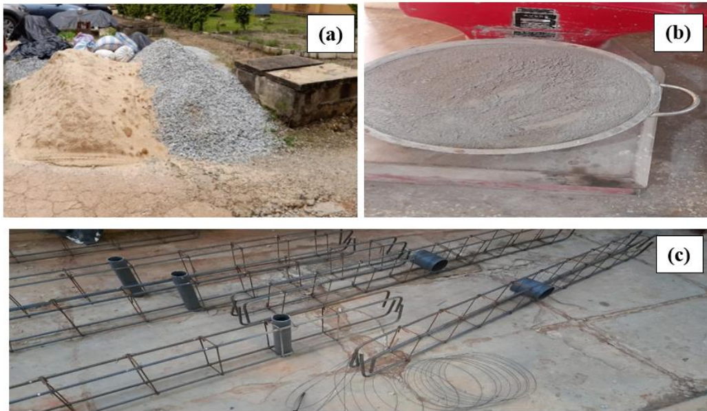
Fig. 1. Materials: (a) sand and gravel, (b) cement, (c) 12mm steel rebars with 8mm stirrups and PVC pipes
